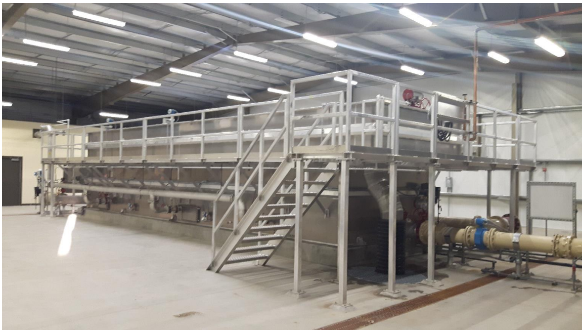
AC Clarifier with Direct Filtration Water Treatment Plant in Apache Junction, Arizona
