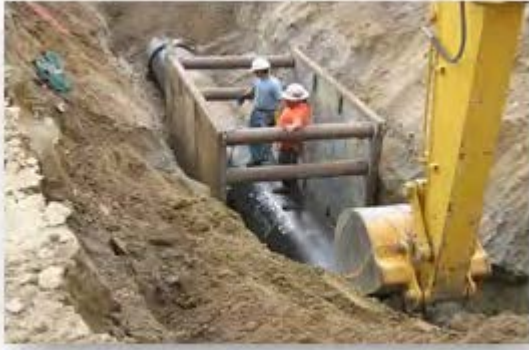
Figure 2. We are proud to have delivered the Ogden Reservoir Pipeline project for SAWCO. Our successful completion of this project created much needed additional capacity and redundancy in SAWCO's water system.
