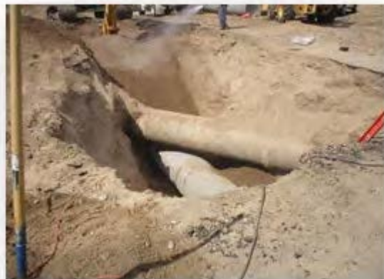
Figure 3. Identification of critical design elements is vitally important to ensure construction changes are
