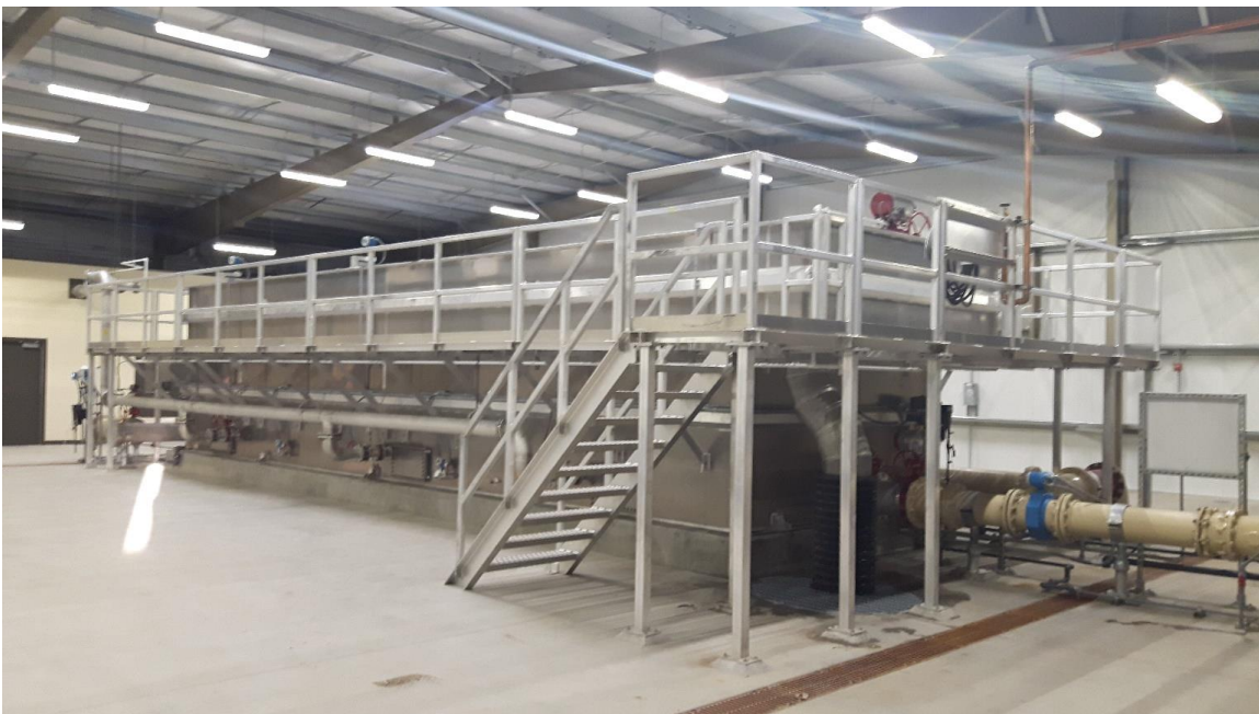
AC Clarifier with Direct Filtration Water Treatment Plant in Apache Junction, Arizona
