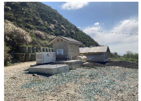
Figure 4 – V-Screen Pump Station.
